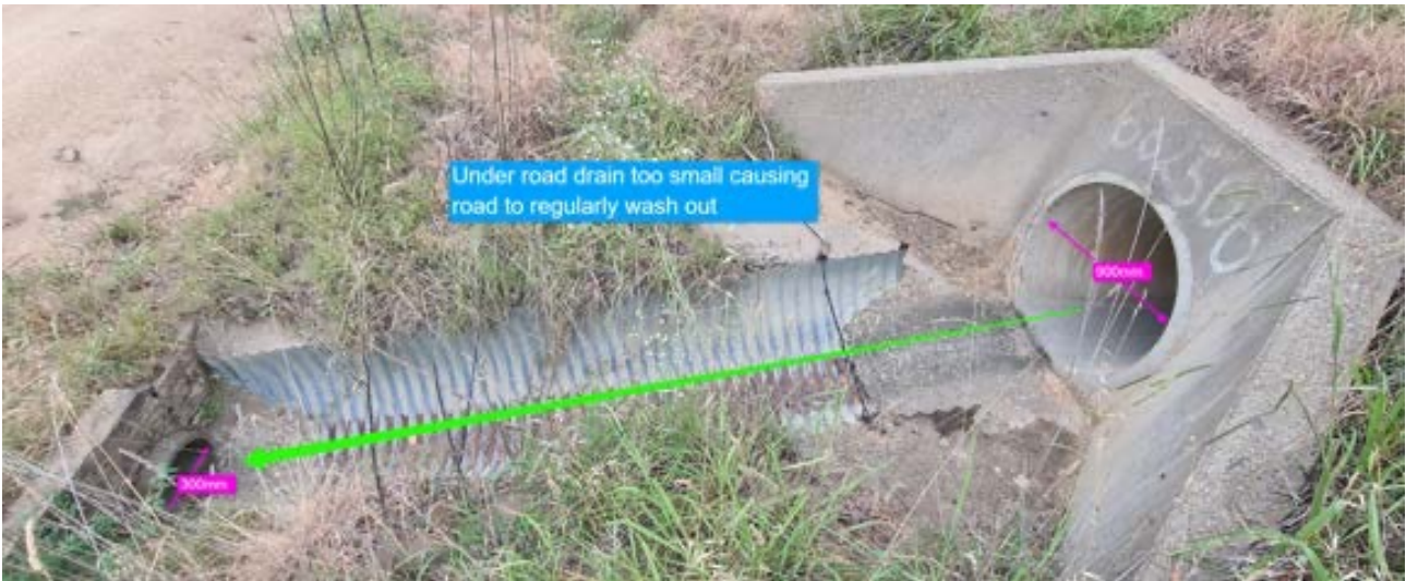
Fig 2. Outflow from Kosci road drain feeds into a drain that is far too small causing storm water to not follow the designed drain path. Drainage system needs to be correctly sized for the catchment.
