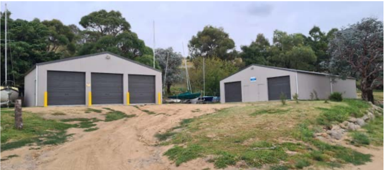
Fig 4. Access roads to boat storage sheds are badly damaged from upstream drainage issues. Multiple attempts to repair the surface with quality materials have been tried, but wash away during heavy rain.
